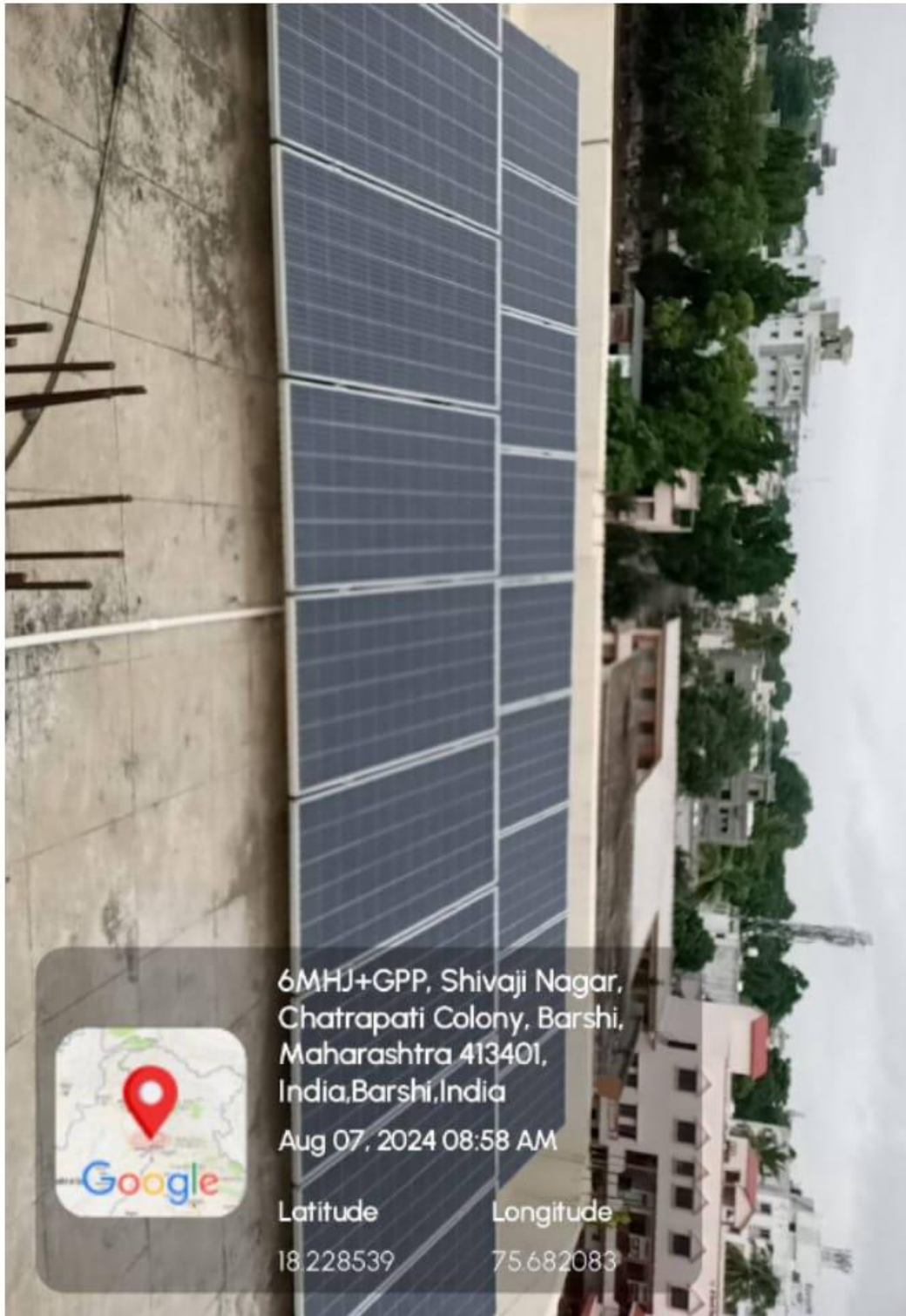
Solar Panels on Library Building
